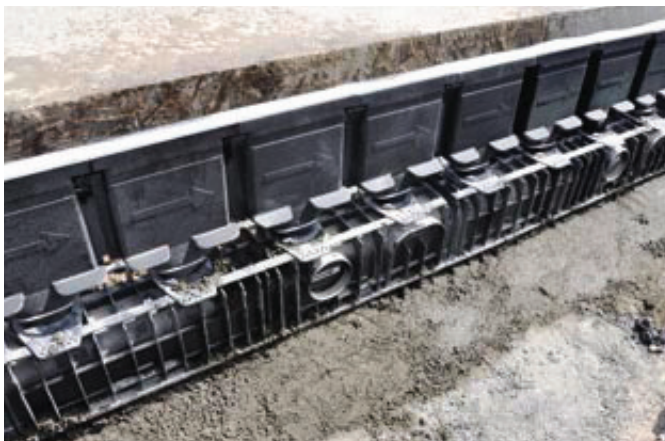
Channel installation at the new Formula 1 track, Yas Marina Circuit, Abu Dhabi
